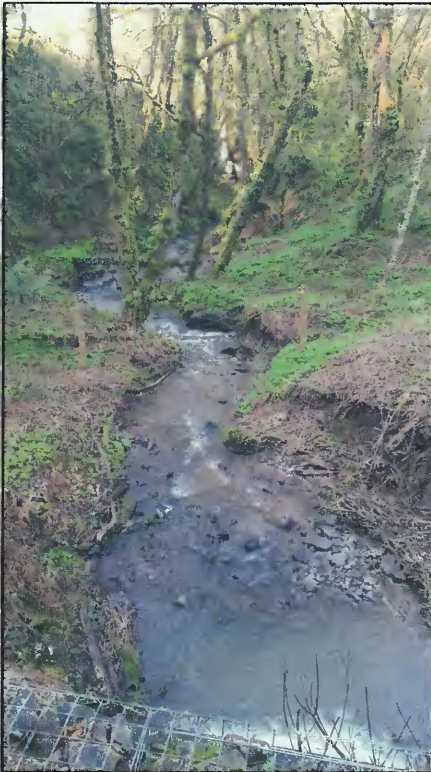
TAKEN ON THE WEST END OF THE ROAD ON TOP OF THE GABION WALL, LOOKING DOWNSTREAM TO THE WEST. (PHOTO TAKEN IN 2015 WITH BRUSH CLEARED. BRUSH HAS GROWN BACK IN 2021 BUT GROUND CONDITION APPEAR UNCHANGED)
