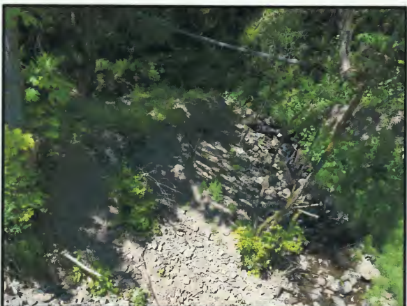
TAKEN ON THE NORTHEASTERLY SIDE OF THE ROAD, LOOKING NORTHEASTERLY UPSTREAM AT THE ROCK AND SOIL DEPOSITS
